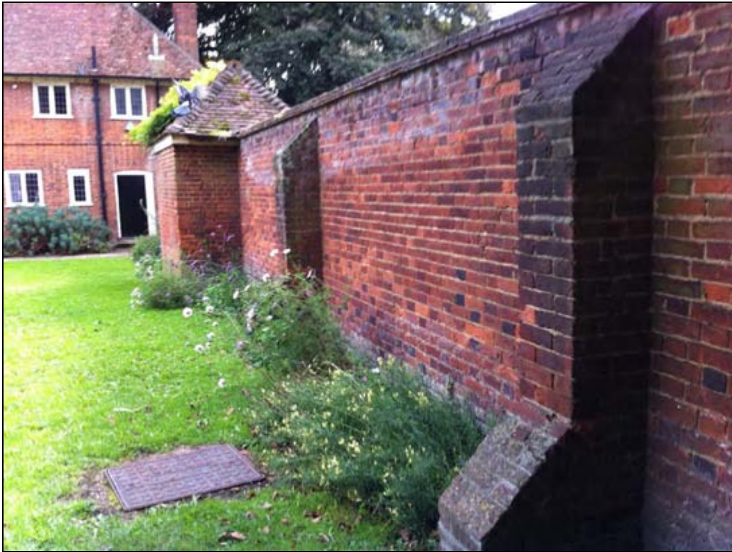
Fig. 23 Part of informal garden, showing Dawber's caretaker cottage, brick wall with buttresses, and shelter. September 2013
